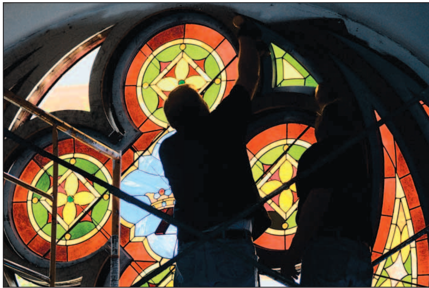
Ken Crisp, left, and Bob Zakas install new stained glass at the former First Congregational Church that is being restored at the corner of M.L. King Boulevard and Lindsay Street.
